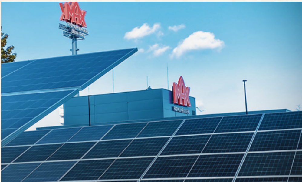
Solar panels on the roof of a MAX restaurant in Poland.
